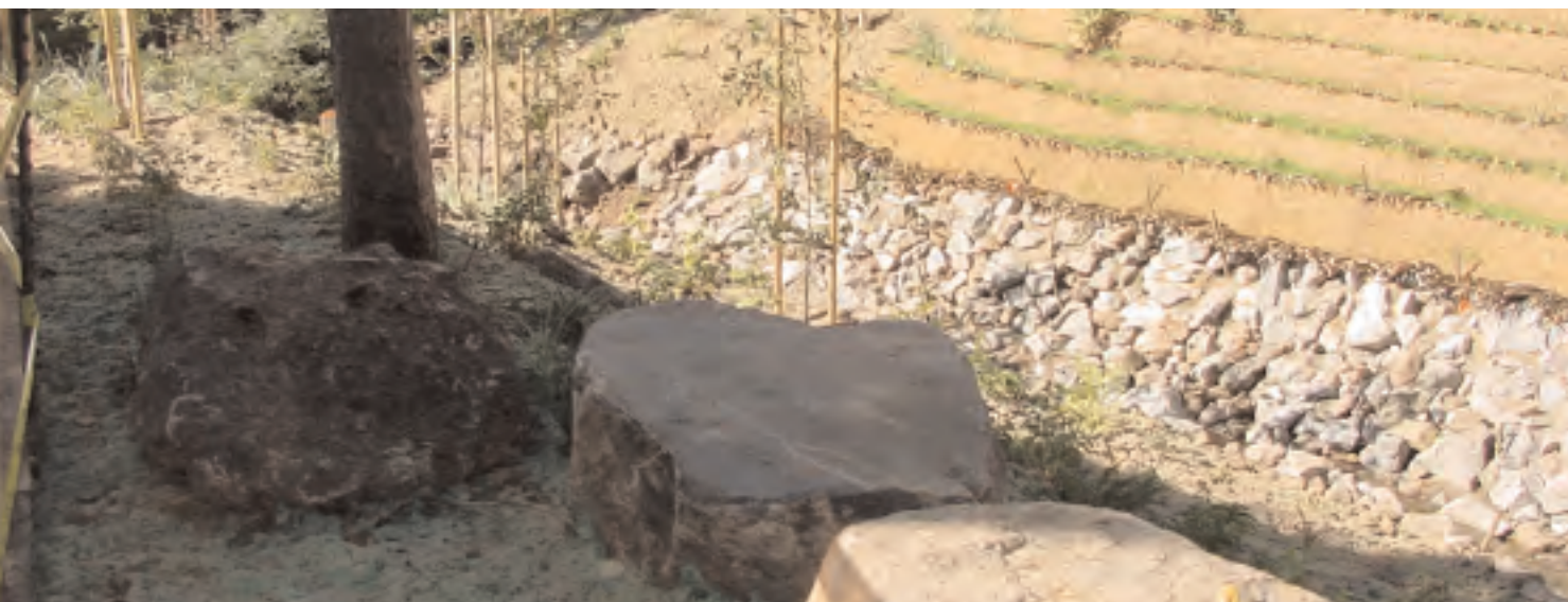
This repaired flood control channel will blend, over time, with the surrounding environment as plantings become established.
