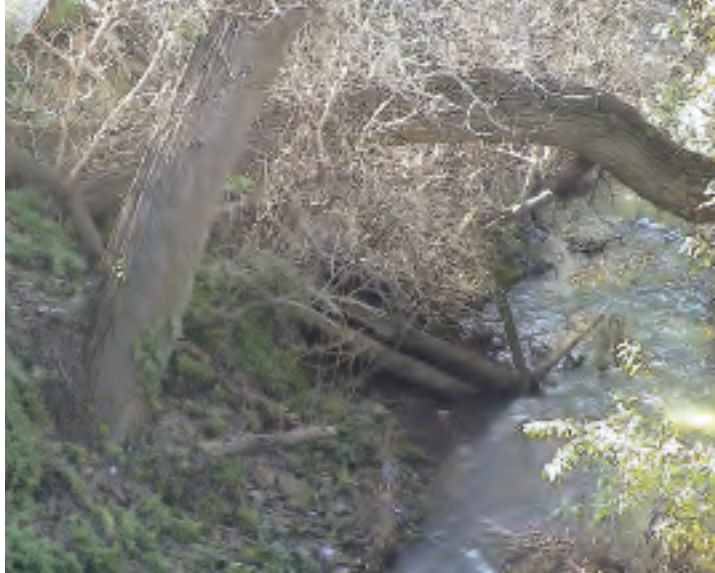
Trees and failed, privately owned retaining walls obstruct this stretch of San Leandro Creek. Future restoration plans include construction to make creek banks less steep, which will minimize future erosion, and replacing invasive vegetation and vines with native plants.
